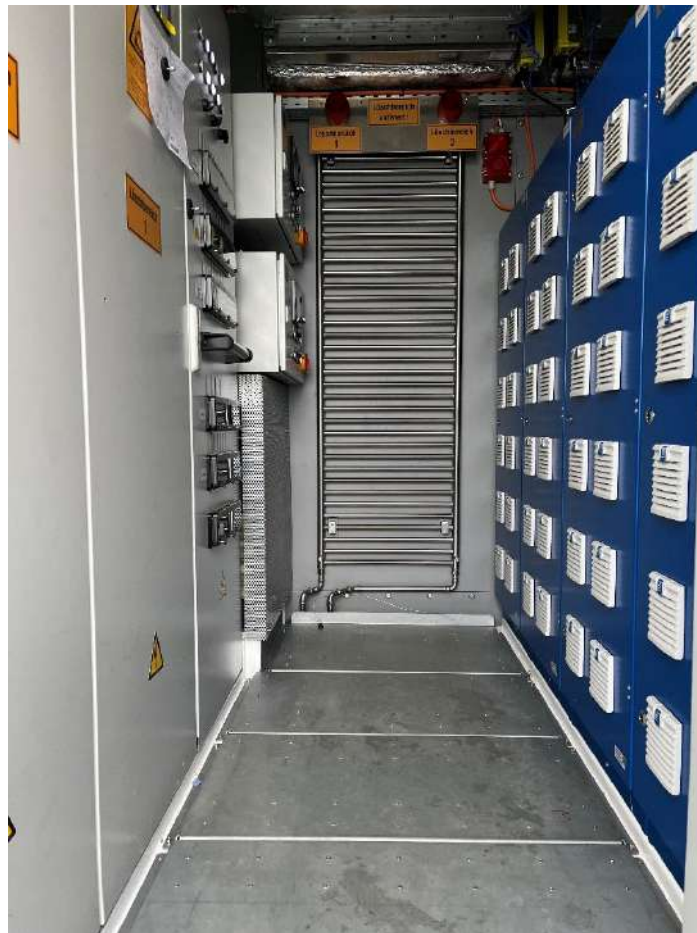
Fig.8: The look into the electrical room of the eCap H2 PowerPac
