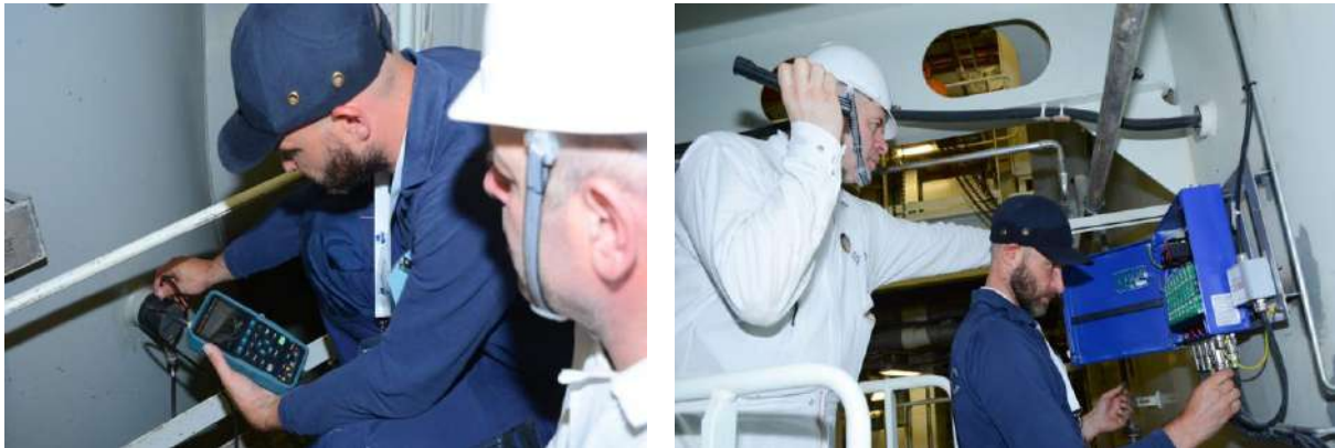
Fig.5: Monitoring of system
